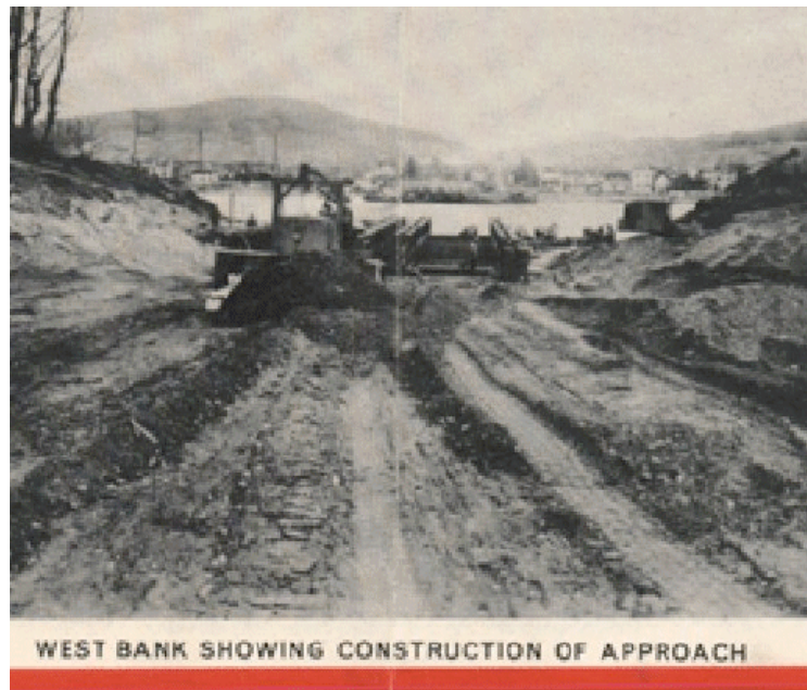
Construction of approach road for the bridge at Bad Godesberg. The vehicle appears to be a tractor. ("Hodges Bridge over the Rhine.")
