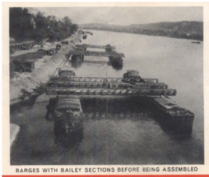
Construction of the Bad Godesberg bridge in sections. (“Hodges Bridge over the Rhine.”)
